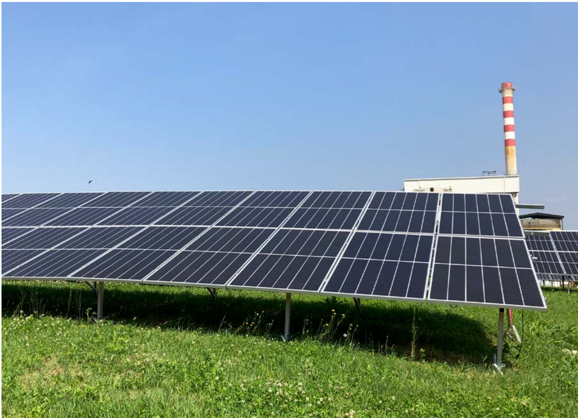
Solar power system at Grünenthal's site in Origgio, Italy
